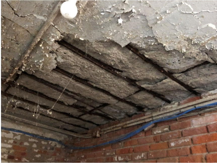
Image 8: Exposed Rebar in Basement
