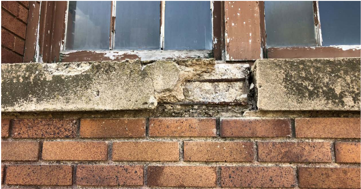
Image 2: Damaged Window and Window Sill
